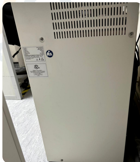
SEPARATE GENERATOR CABINET
